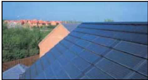
Figure 10 – Typical Domestic PV Installation
