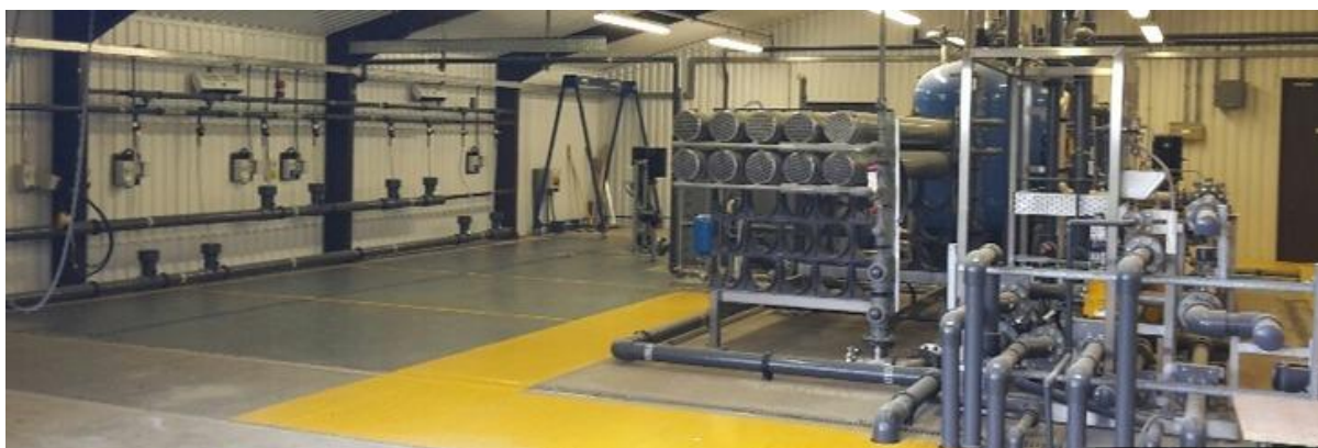
Figure 6: Gorthleck Development Centre (Courtesy Scottish Water)
