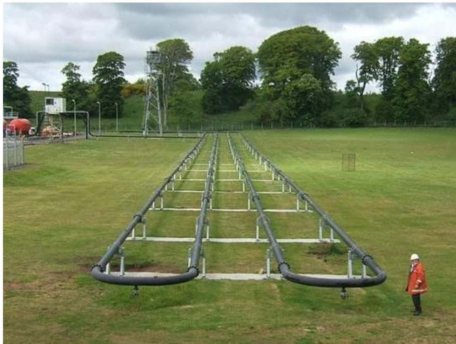
Figure 9: Petrofac’s 1km 10” pipe test rig at Montrose
