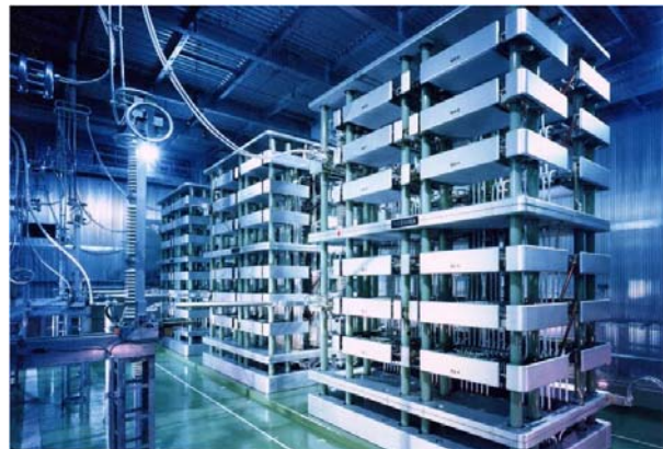
Figure 2: 700MW, 250kV HVDC converter station installed in Japan
